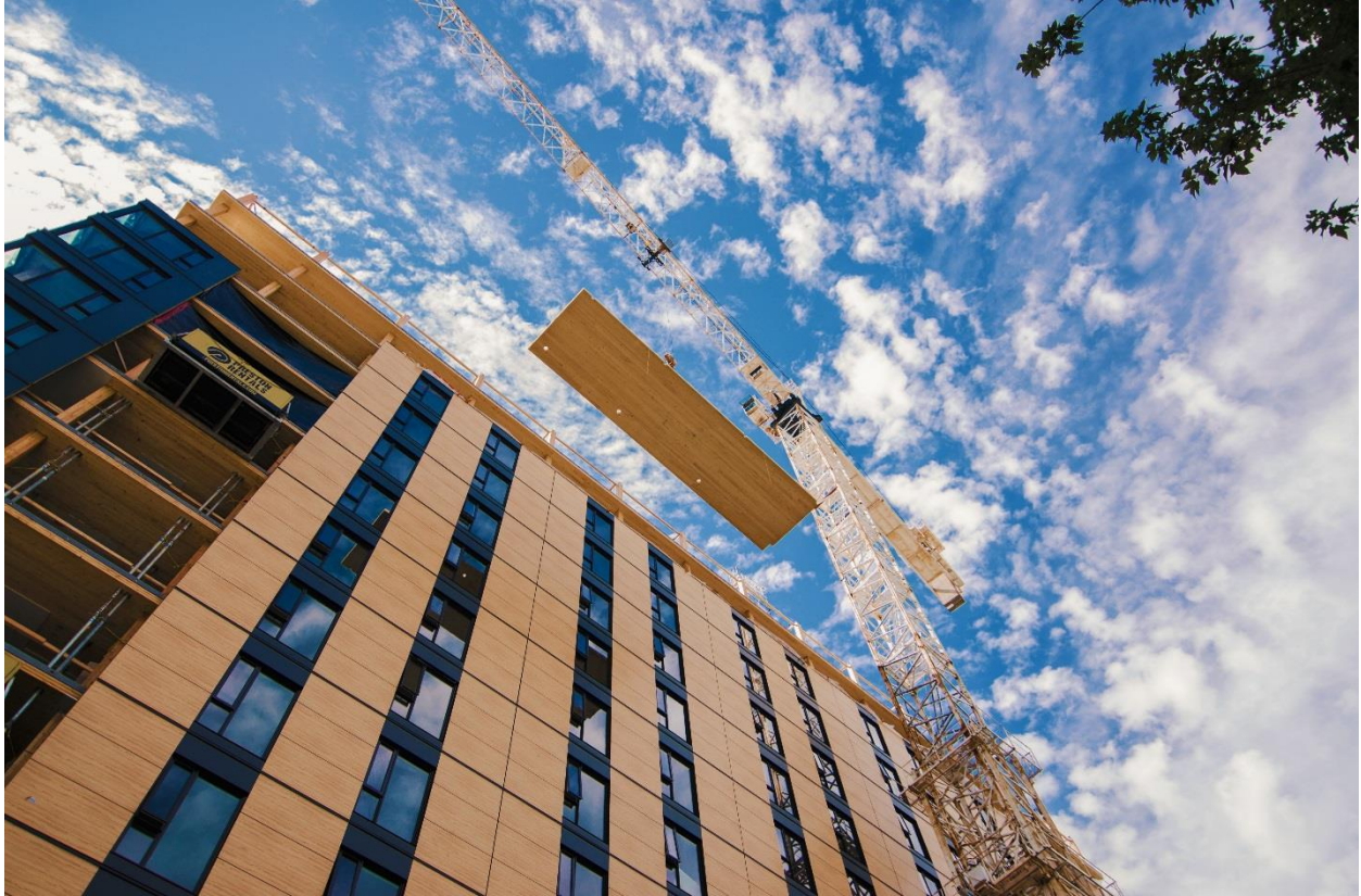
Figure 1: Brock Commons at the University of British Columbia – the world's tallest wood building. Courtesy of Seagate Structures.
